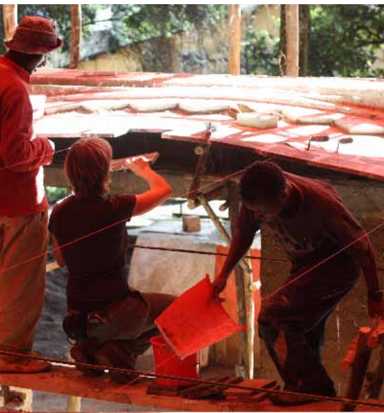
Sustainable Urban Dwelling Unit (SUDU) under construction – building with low cost material, local resources and the capacity of daily labourers.
